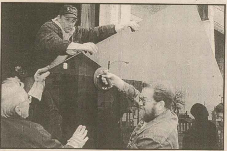
Heavy Lifting - Workman install a new 500 pound window at La Cage. The 2 inch thick, tempered, thermal pane smoked glass is one of two windows being put in outside of the Dance Dance Dance area. Raised seating areas with tables and chairs will be next to the windows providing patrons with a view of the busy Second Street bar area.
