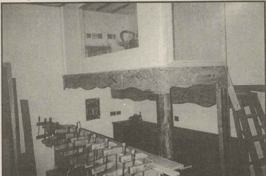
Sprucing It Up - The picture above shows some of the work being done at Fannies, 200 E Washington as the bar prepares for its grand reopening on Saturday March 14. The popular Lesbian hot spot was destroyed by a fire last year. Shown above are work on a new second bar and the new DJ booth.
