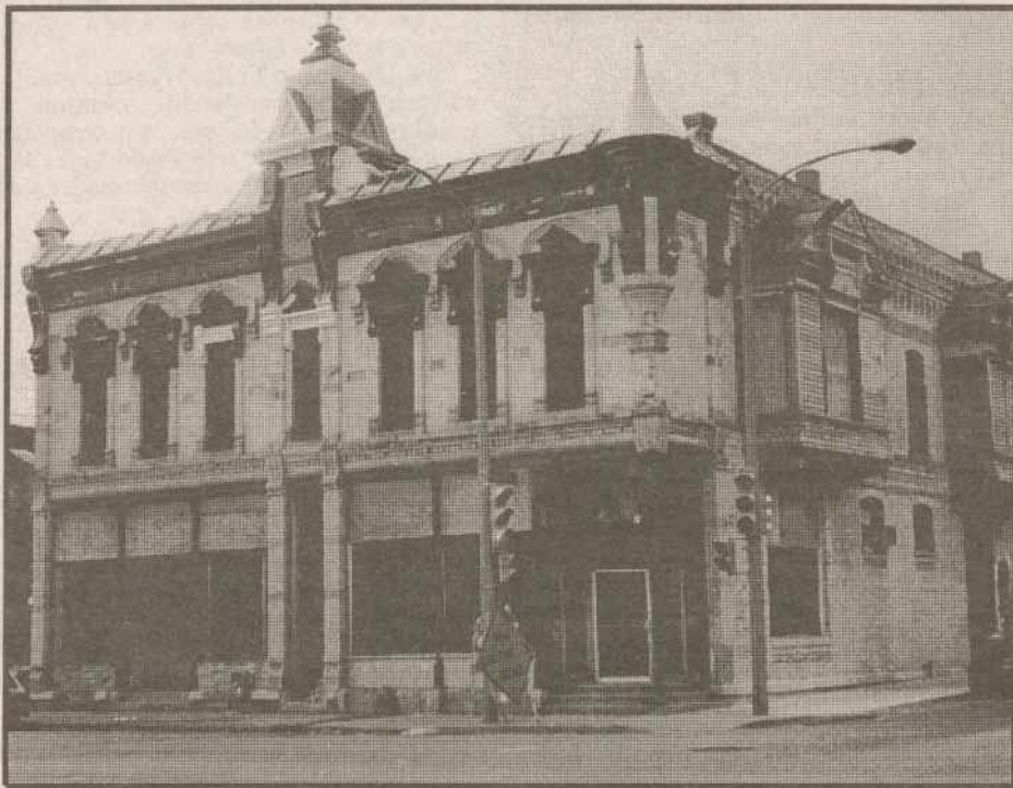
New Old Look — As you can see from this picture, the work on restoring the exterior of La Cage in Milwaukee to its original look is going well. The bricks have been chemically cleaned for their paint revealing the splendid cream city brick look. The windows are also being restored to their original look. Plans for interior remodeling are also well underway.
