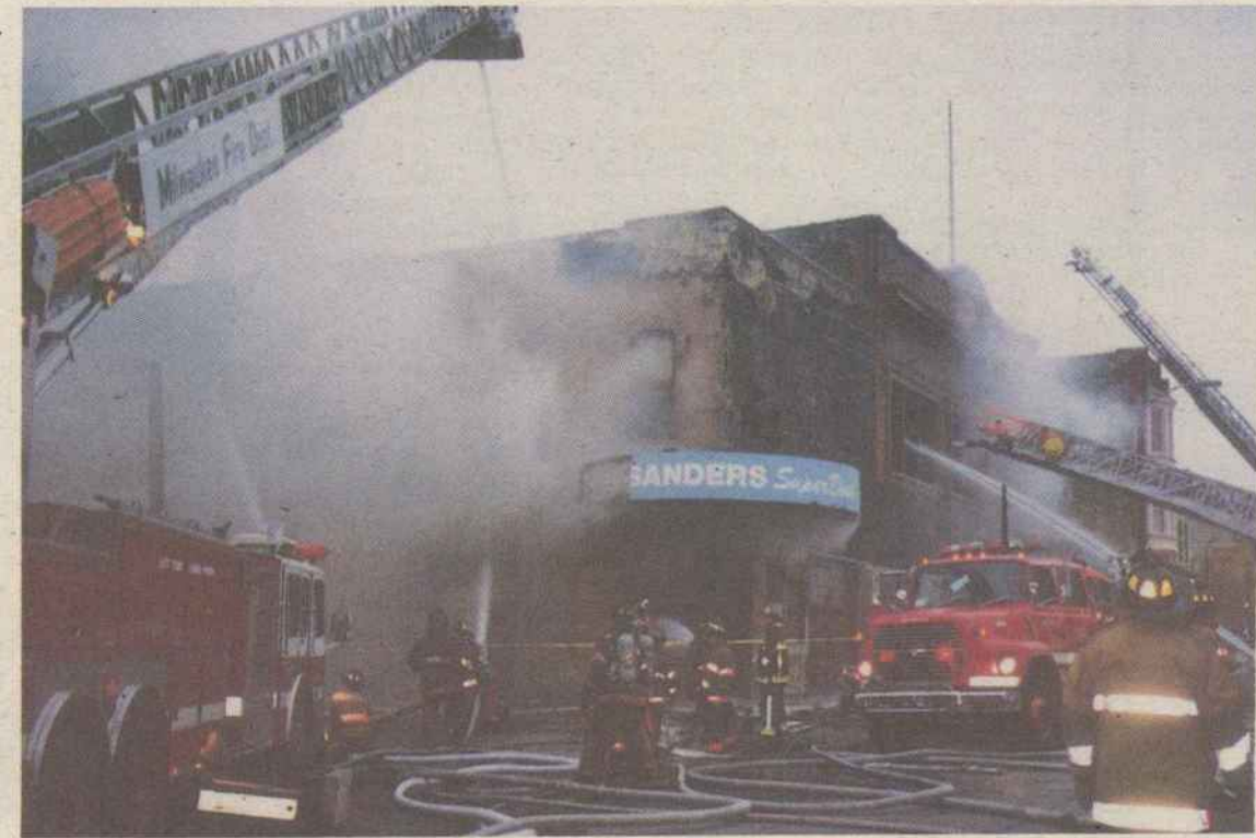
Fire at the Community Center - A three alarm blaze at the site of Milwaukee's new LGBT Community Center filled the neighborhood with smoke. The fire was accidentally started by a worker using a welding torch. More pictures of the fire and inside damage are on page 6.
