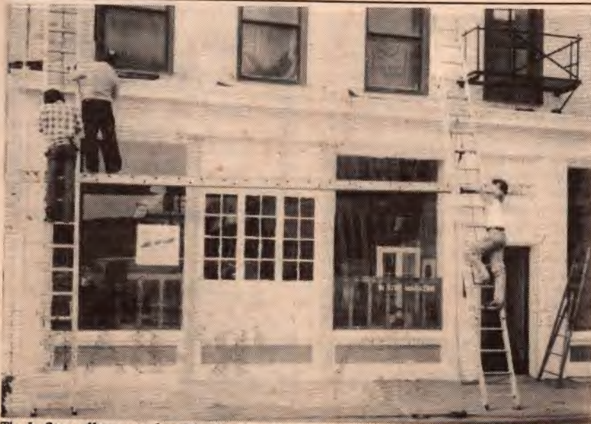
The In Step office got a face lift with a bright white and shades of grey paint job. The Cream City Foundation will be moving into the other half of the building soon.
